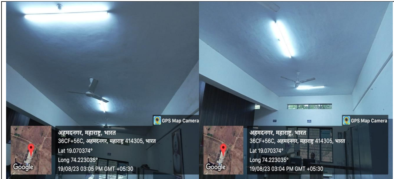
LED Tubes in the Office
