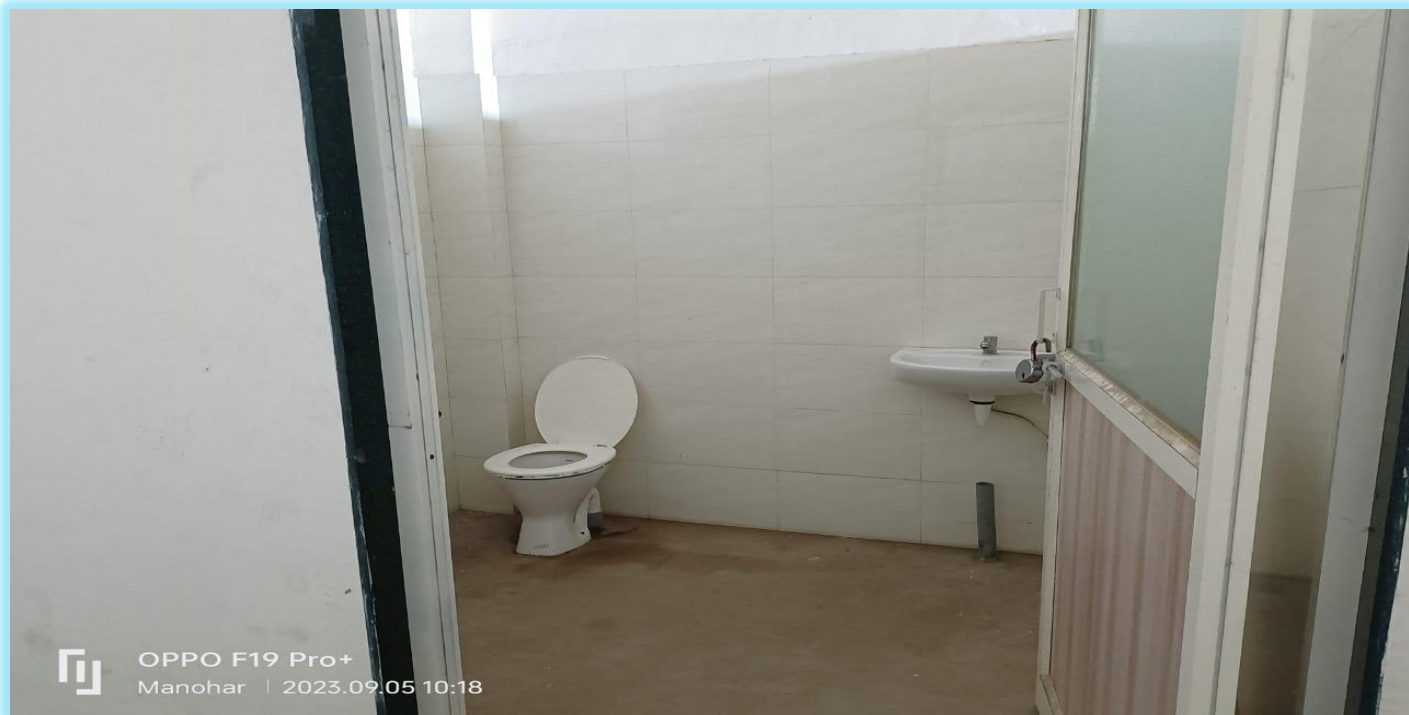
WASH ROOM FOR HANDICAP
